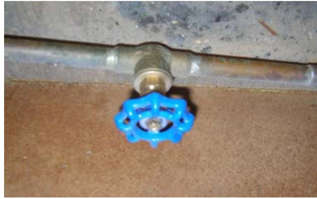
zone shut-off valve
