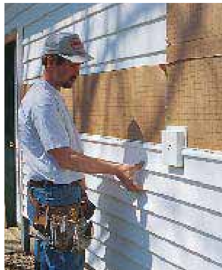
Figure 6. Subcontractors can create problems when they fasten exterior fixtures directly through the siding panels, because the fasteners will prevent the siding panels from expanding and contracting freely. Use mounting blocks for all surface-mounted fixtures.
